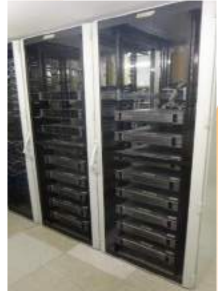
RBC Test Bench hardware installed in a cabinet together with tested equipment
